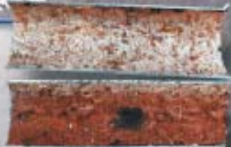
General Pipe Deposit
