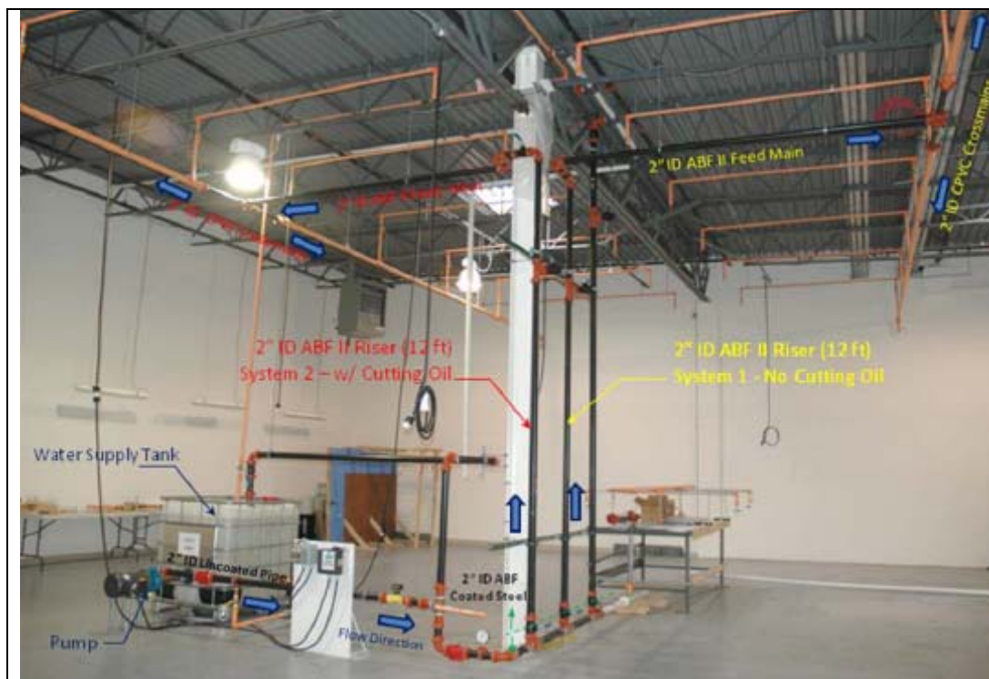
Figure 2. Photograph of a portion of the intermediate scale system, including the reservoir, pump, riser, and crossmains.
